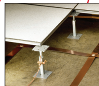
Signal Reference Grid (SRG)
